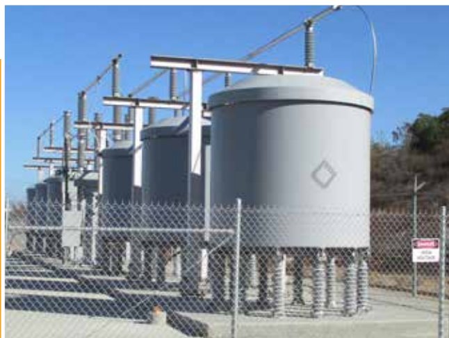
69 kV Shunt Reactors (USA)
